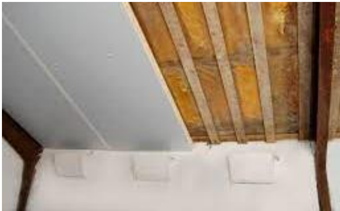
Figure 1: Ceiling insulation of old pig stable using polyisocyanurat (PIR) (source: Recticel Insulation)
